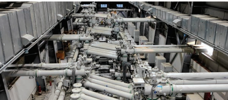
400kV GIS Switchyard at BIFPCL's 2x660MW Maitree TPS in Bangladesh
