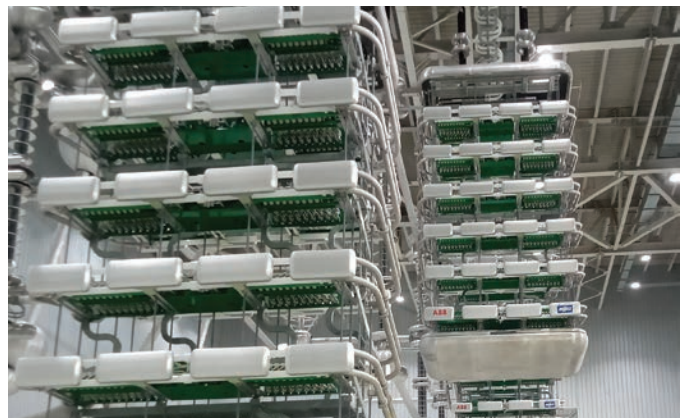
Valve Hall at Raigarh HVDC Converter Station
