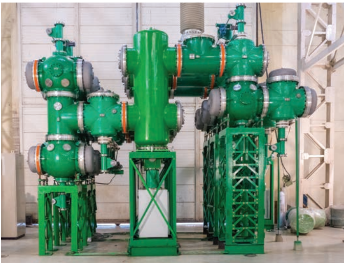
400 kV GIS for Chamera HEP
