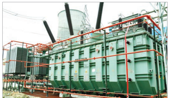
India's first 400 kV Phase Shifting Transformer
