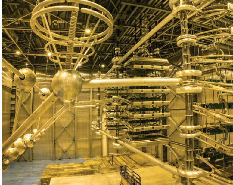
Indoor DC Hall at NE Agra HVDC Terminal
