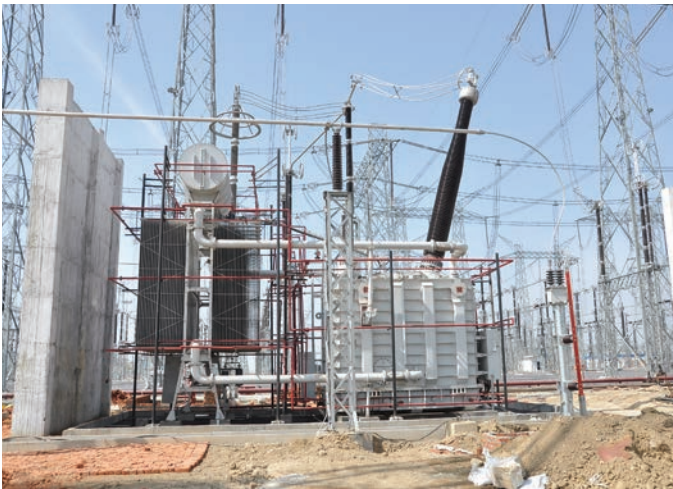
India's first 400 kV Controlled Shunt Reactor at Itarsi Substation
