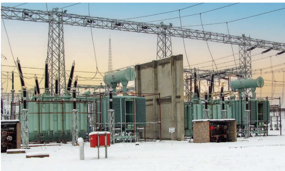
220/ 20 kV substation at Charikar, near Kabul, Afghanistan
